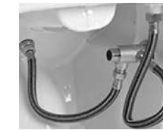
Bidet inlet pipe
